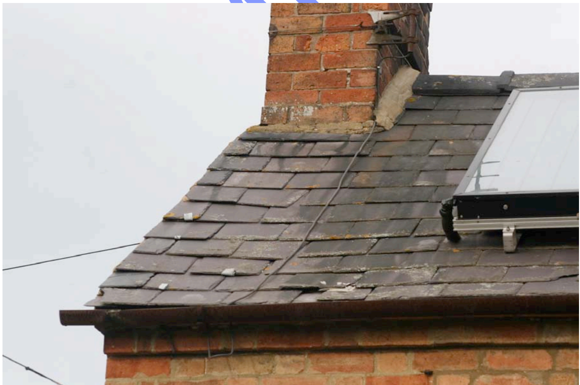
PHOTOGRAPH NO. 6 Broken and repaired slates on rear roof
