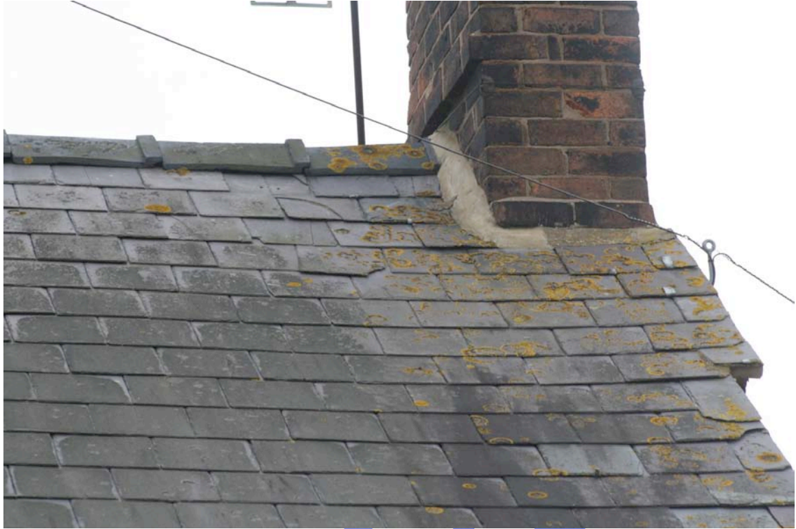
PHOTOGRAPH NO. 3 Broken slates on front roof
