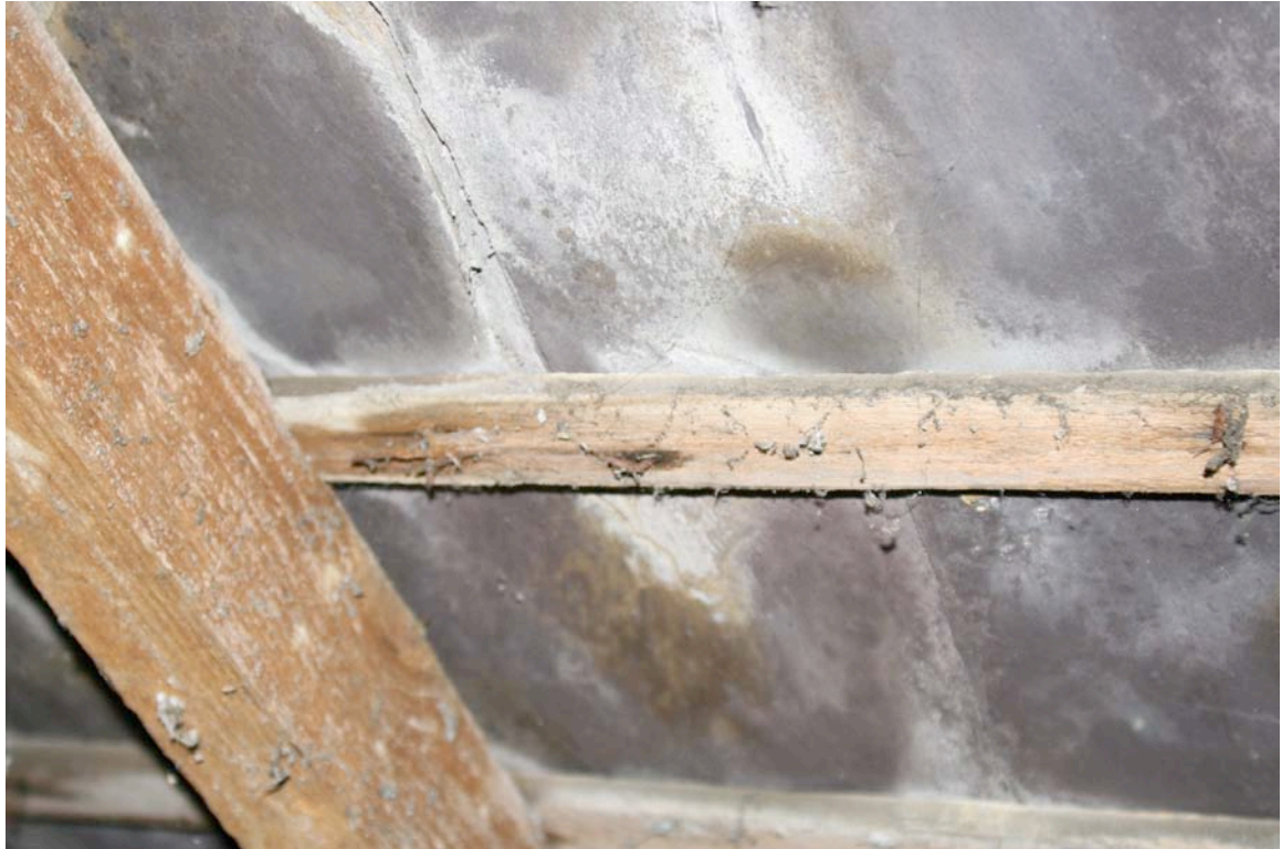
PHOTOGRAPH NO. 7 Taken in roof space - rusty nails fixing slates
