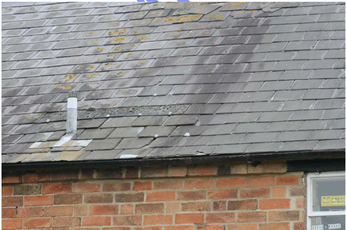
PHOTOGRAPH NO. 4 Broken slates on front roof
