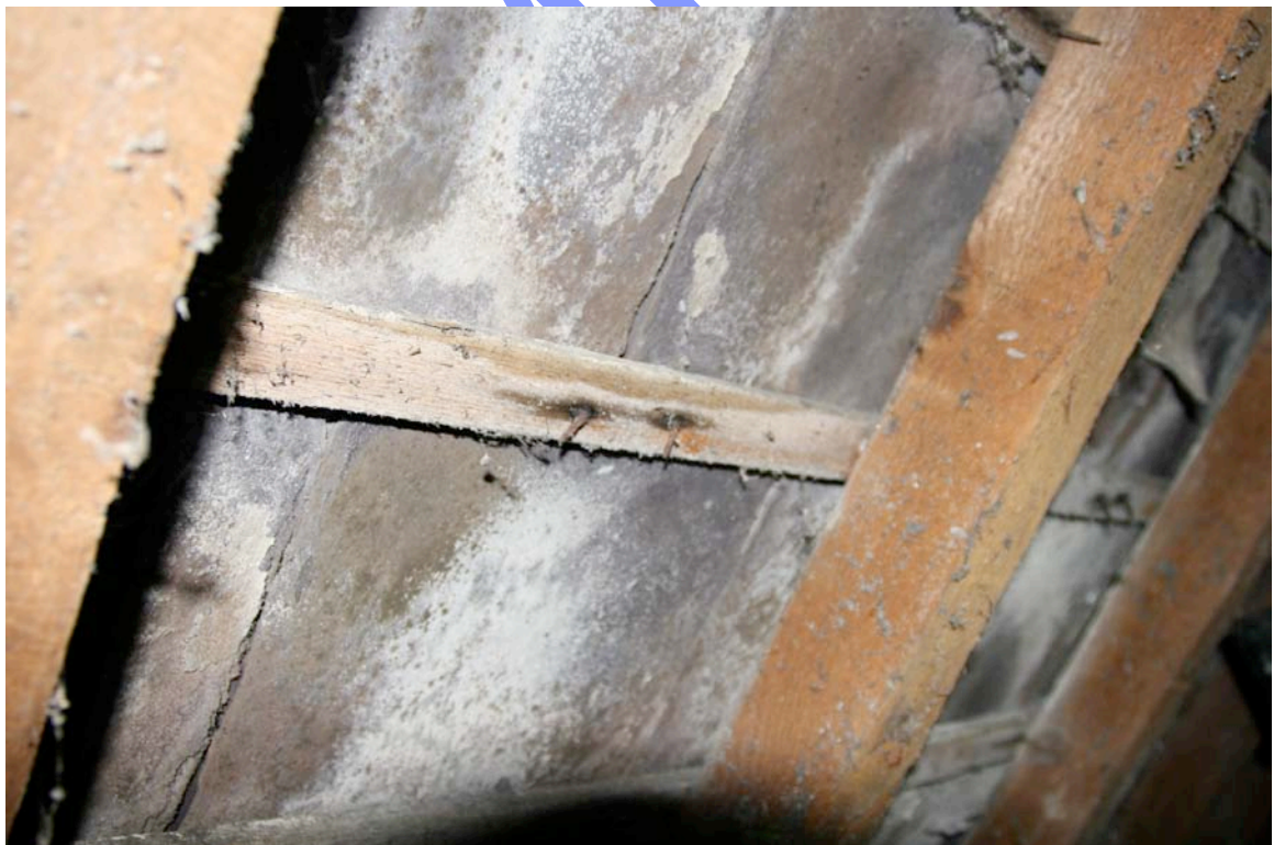
PHOTOGRAPH NO. 8 Taken in roof space - rusty nails fixing slates
