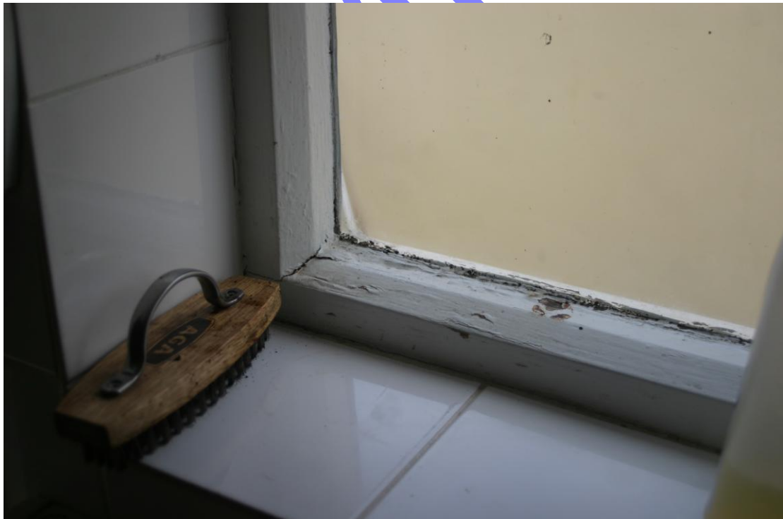
Photograph No. 217. Rot inside the kitchen window frame
