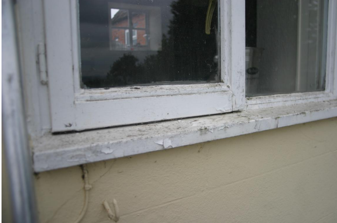
Photograph No. 215. Paint peeling from landing window
