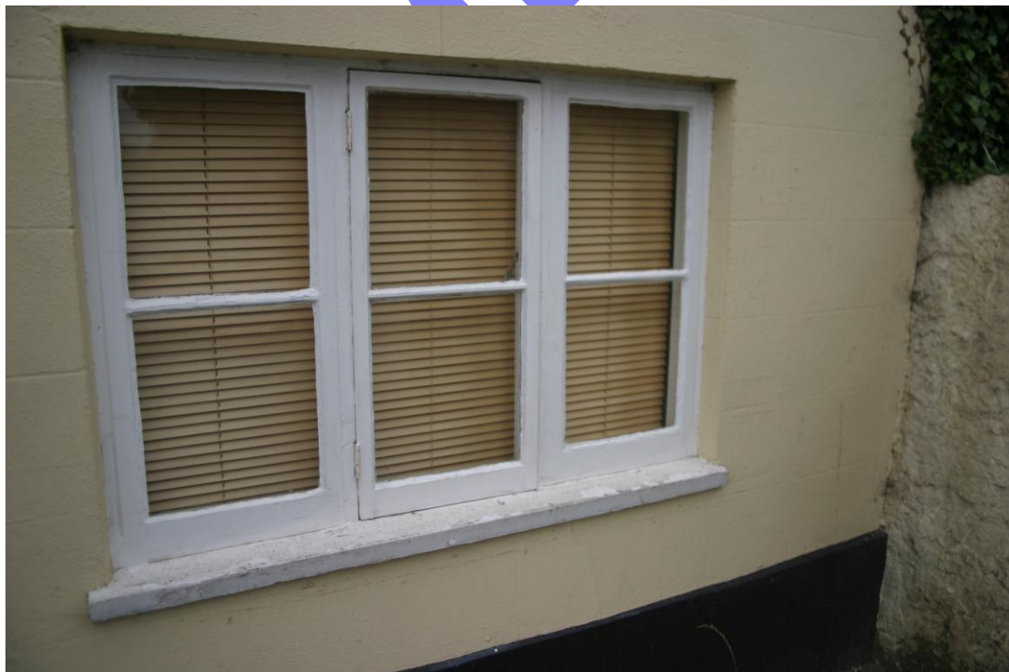
Photograph No. 212. Paint peeling from lounge bar window
