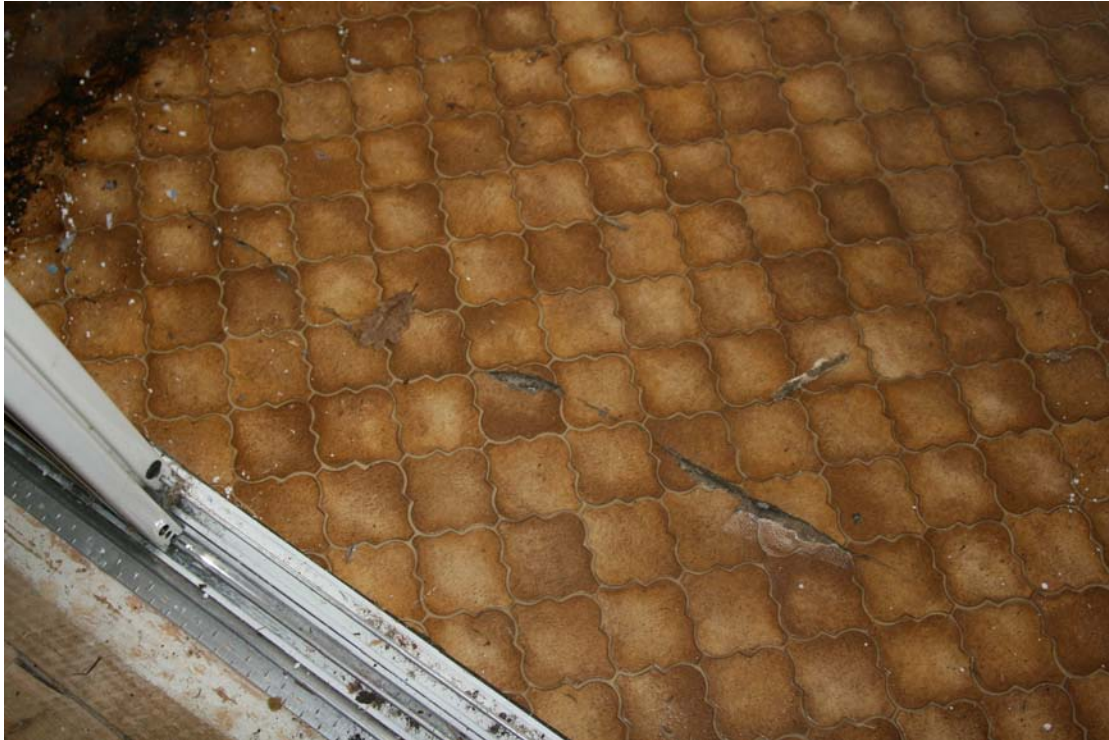
PHOTOGRAPH No. 13 - crack across kitchen floor
