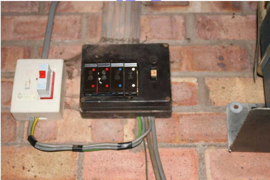
PHOTOGRAPH No. 77 - The electricity fuse board
