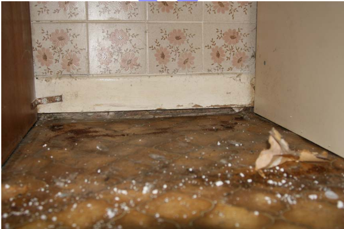
PHOTOGRAPH No. 14 - gaps between skirting and kitchen floor
