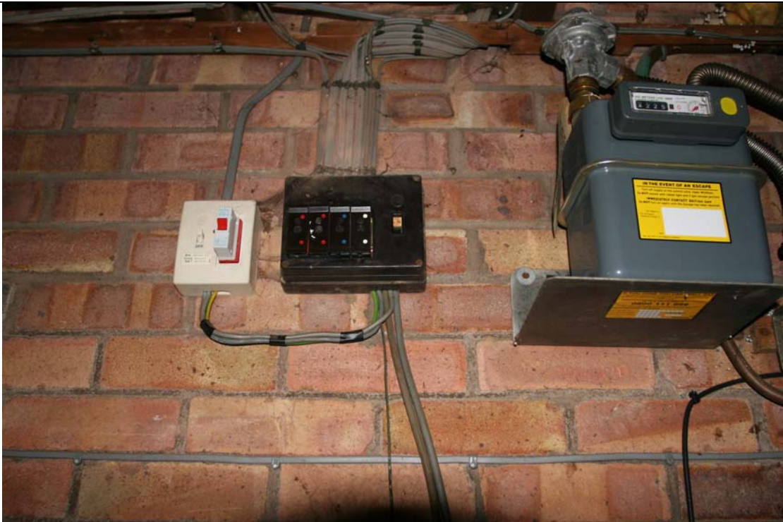
PHOTOGRAPH No. 76 - The electricity fuse board
