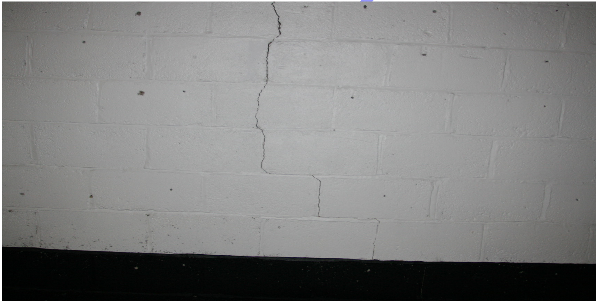
PHOTO No. 410 CRACK THROUGH THE LEFT HAND WALL INTERNALLY
