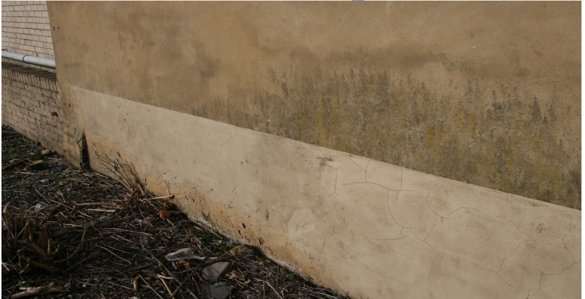
PHOTO No. 411 CRACK THROUGH THE LEFT HAND WALL INTERNALLY
