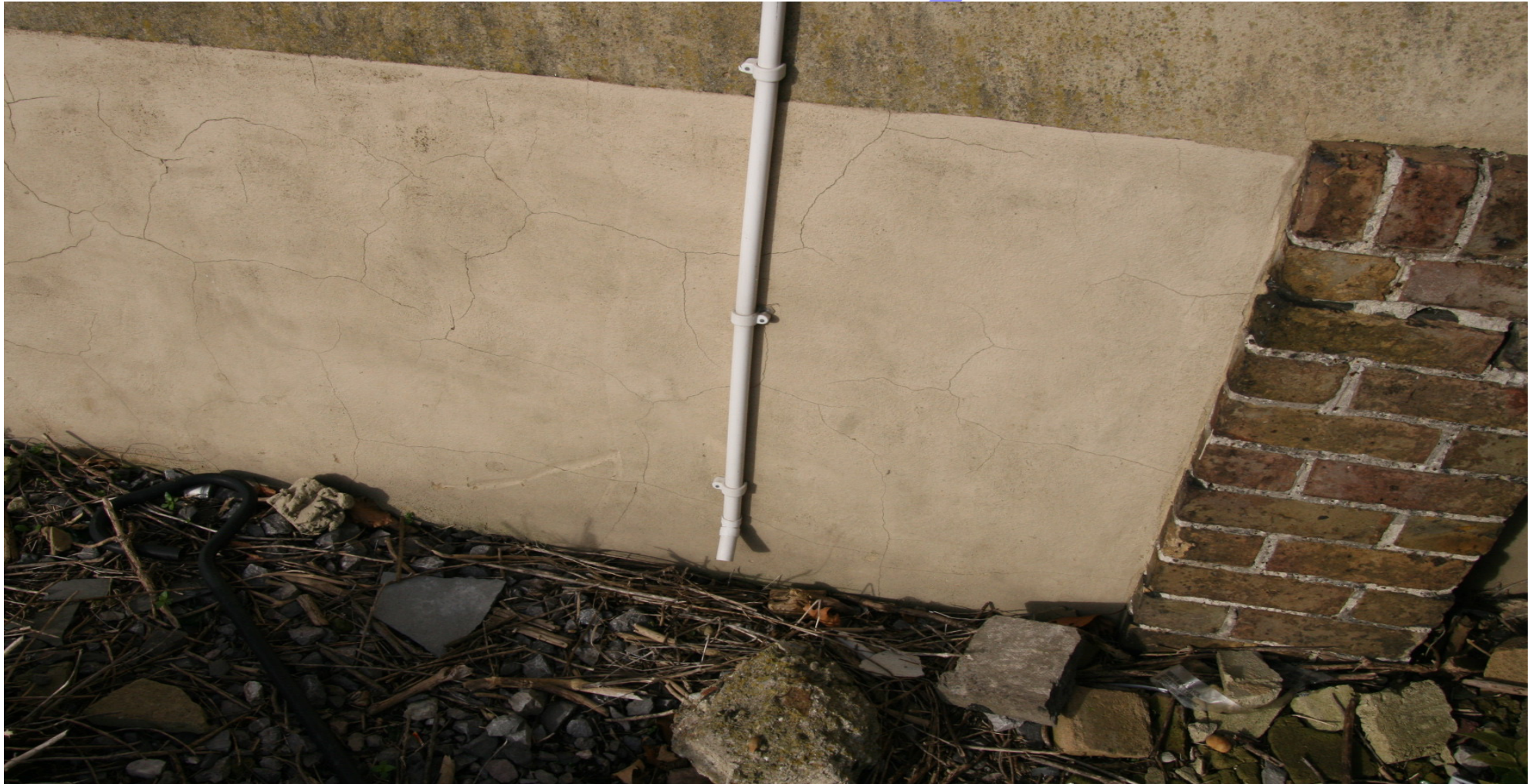
PHOTO No. 263 CRAZED AND LOOSE RENDER ON THE LEFT HAND WALL EXTERNALLY
