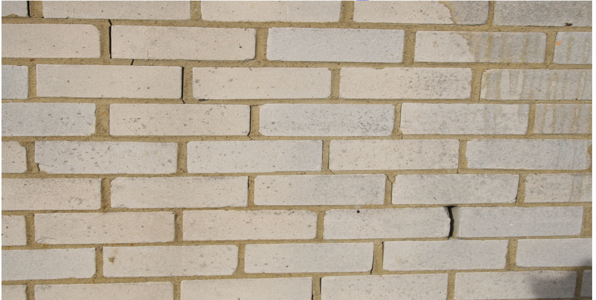
PHOTO No. 240 CRACK THROUGH THE LEFT HAND WALL EXTERNALLY
