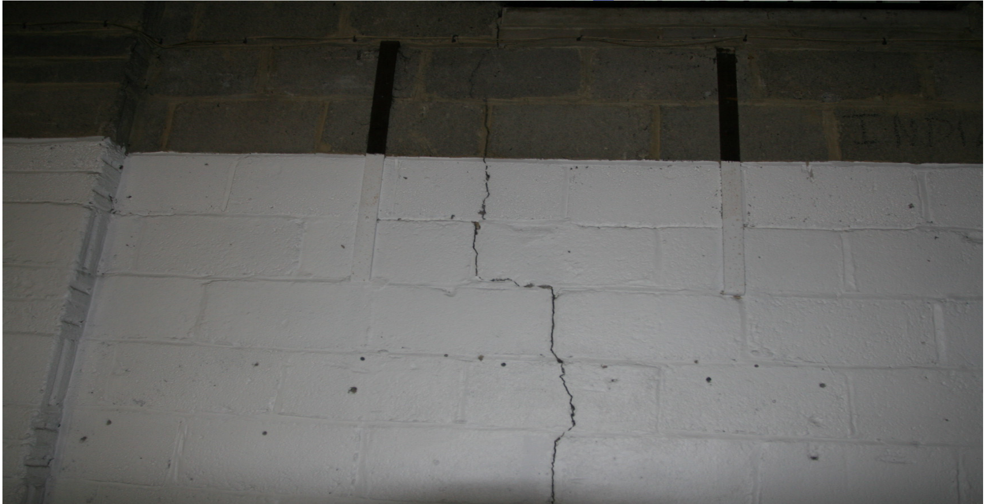
PHOTO No. 241 CRACK THROUGH THE LEFT HAND WALL EXTERNALLY
