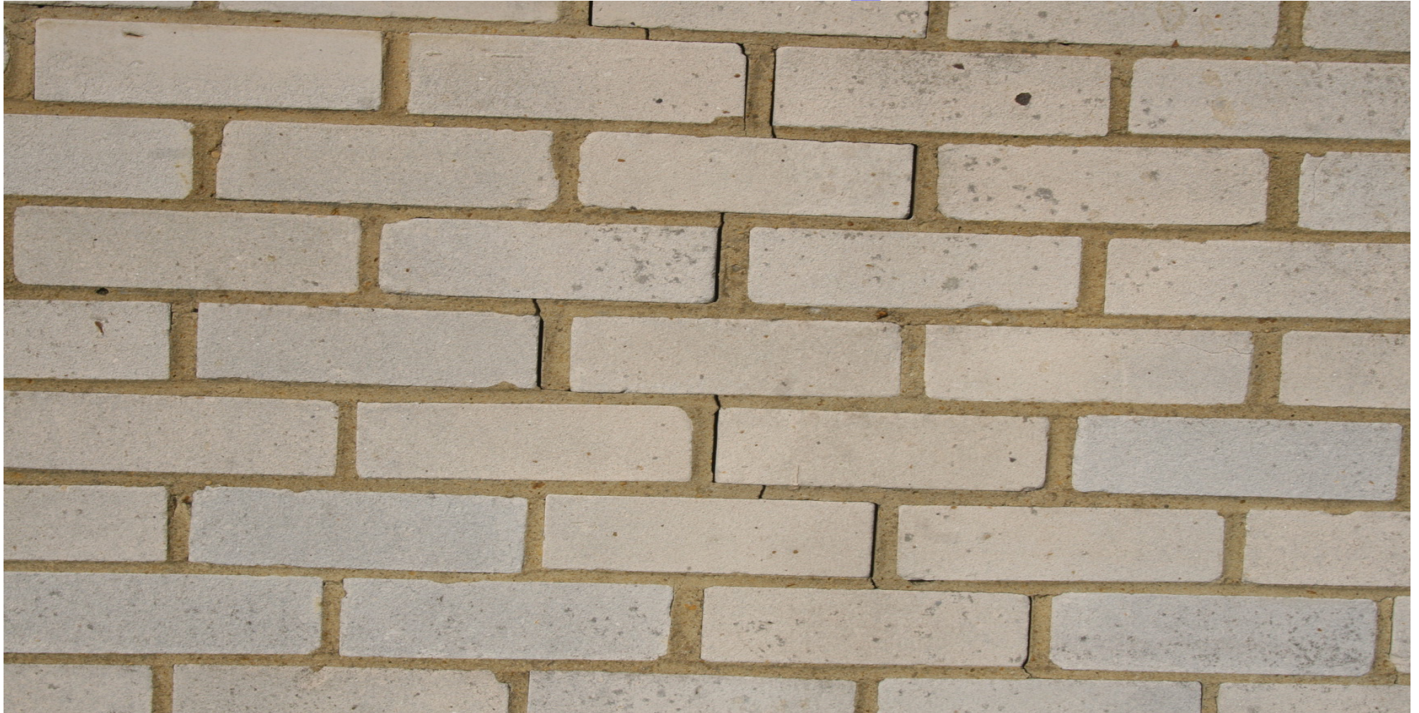
PHOTO No. 239 CRACK THROUGH THE LEFT HAND WALL EXTERNALLY
