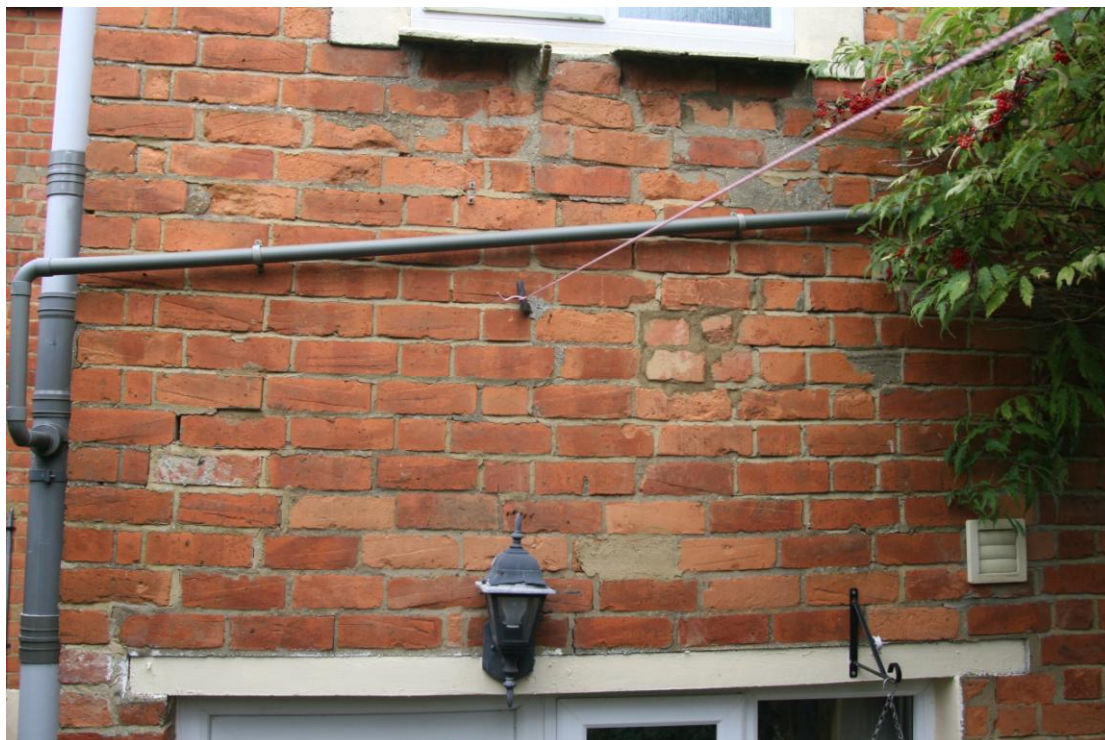
PHOTOGRAPH No. 20 - Distortion above the kitchen window
