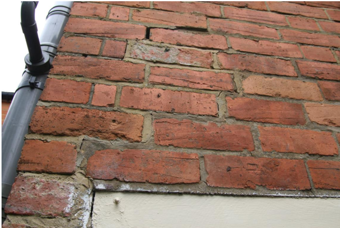
PHOTOGRAPH No. 24 - Cracking above the kitchen window/door
