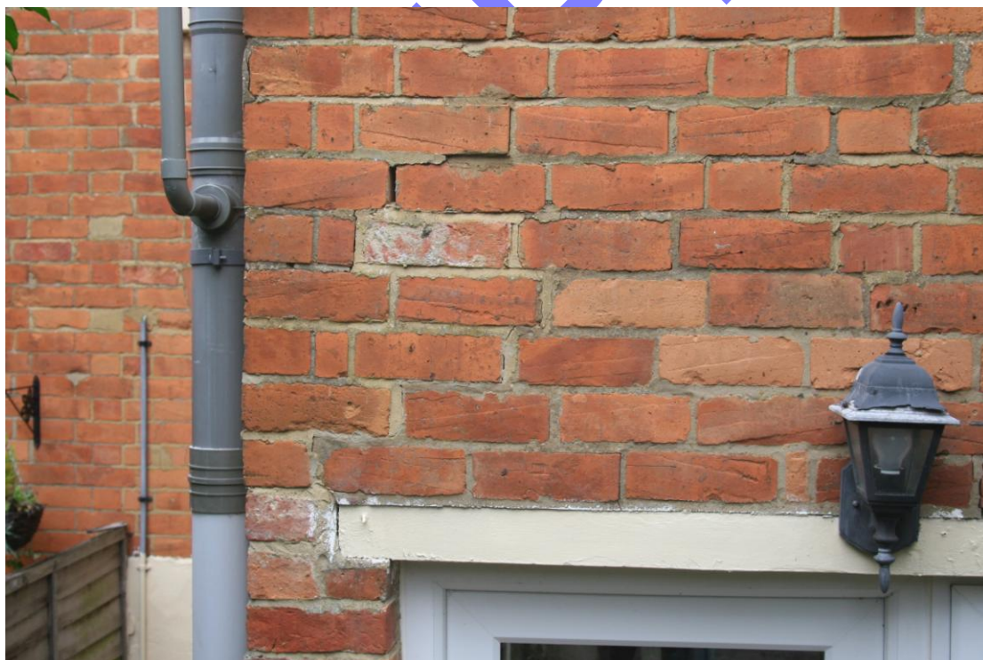
PHOTOGRAPH No. 22 - Cracking above the kitchen window/door
