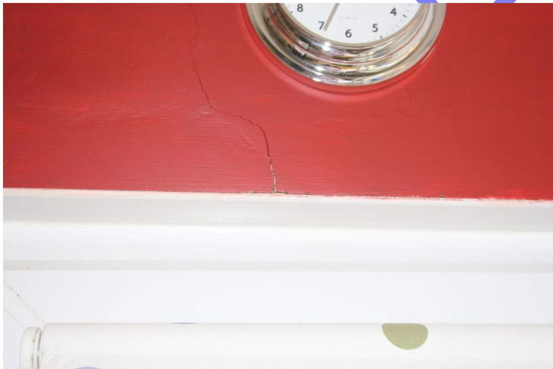
PHOTOGRAPH No. 41 - Plaster crack above the kitchen door
