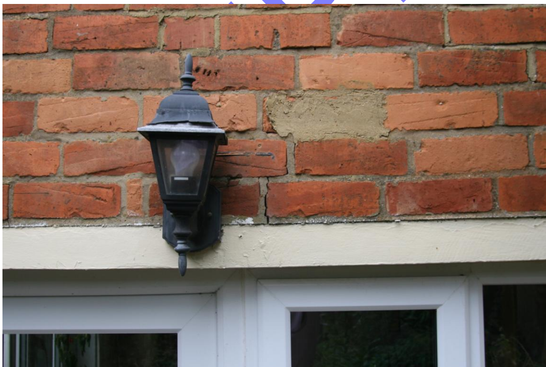
PHOTOGRAPH No. 25 - Cracking above the kitchen window/door
